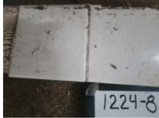
1224-8 Ceramic Tile/Grout Interior Bathroom
